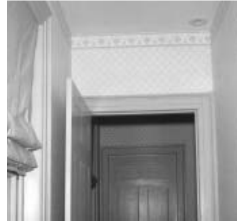
A Unico System outlet provides modern day comfort without marring the original aesthetics of the Daniel Wheaton Home, c. 1796
