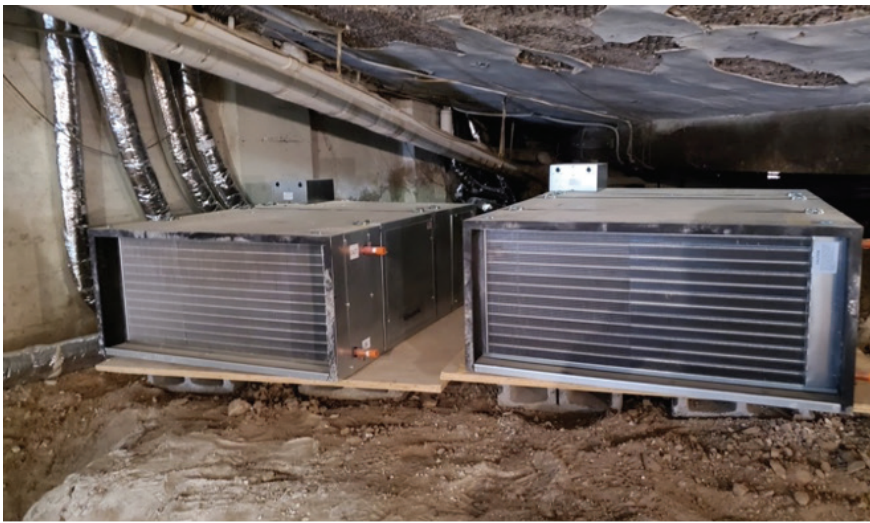
Two of the four Unico air handlers located in the basement. All are equipped with hot water coils for heating.
