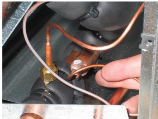
Figure 29. Thermal Measuring Bulb Placed on Copper Tube.
